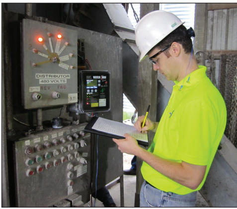
Brian Knapp, 4B Components vice president of technical sales and service-Electronics Division, performing a Tech Team inspection on a Watchdog Super Elite monitoring system.
