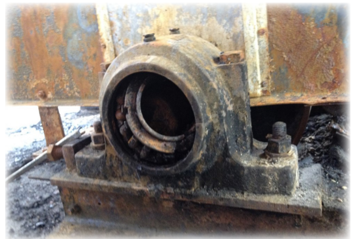
Image 2: Faulty bearing ; cause of fire
