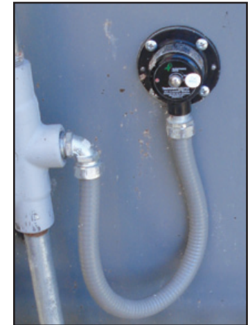
Touchswitch installed on a bucket elevator
