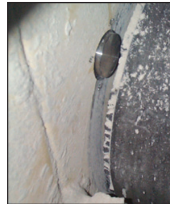
Touchswitch installed at the drive end of an enclosed belt conveyor (inside view)
