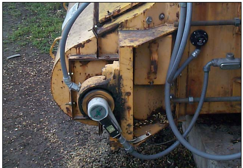
Whirligig installed on an enclosed belt conveyor shown with M800 speedswitch
