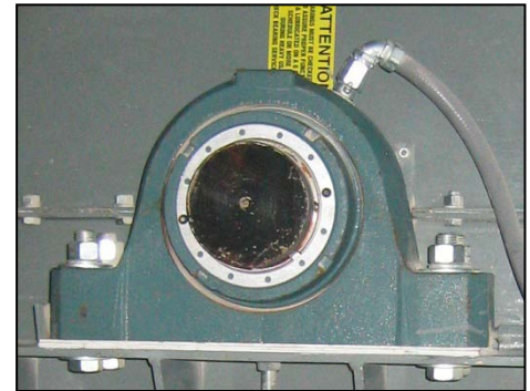
Sensor Installed on Conveyor Bearing
