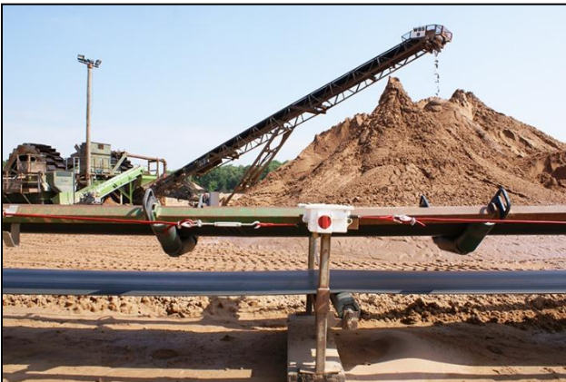
Pullswitch Installed on Open Conveyor at Sand and Gravel Facility
