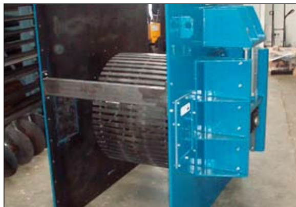
Replace dust-free elevator boot.
